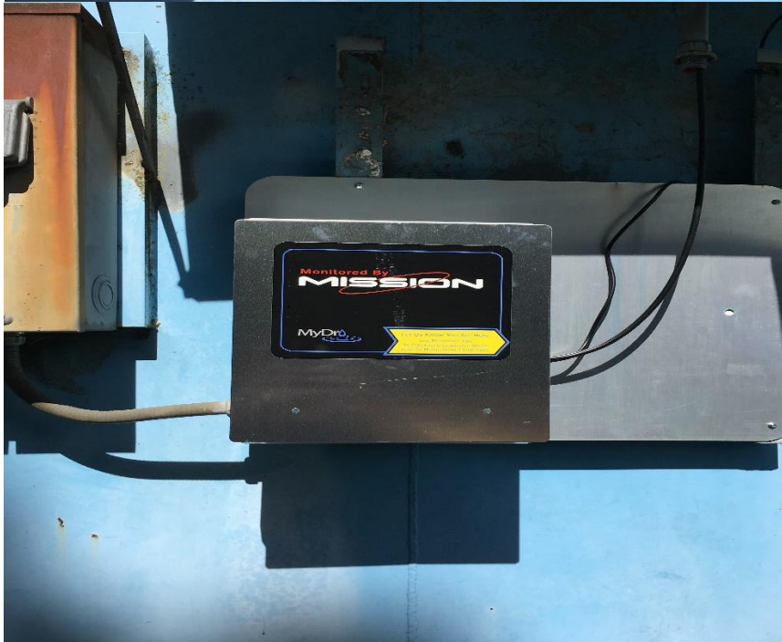
New Mission Communication with Battery Backup
